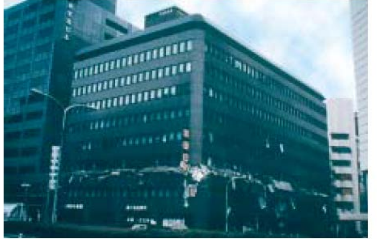
5/1 In this commercial building the third floor has disappeared and the floors above have collapsed onto it (Kobe, Japan 1995).
